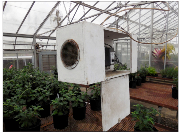
Figure 12. Aspirator box to house thermostats.
